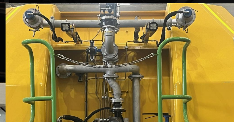
RF WATER CONTROL
